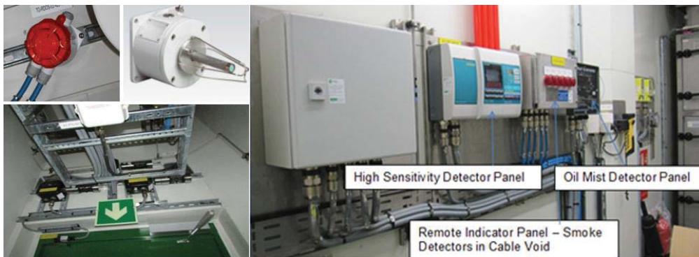
Safety Systems – Detection
