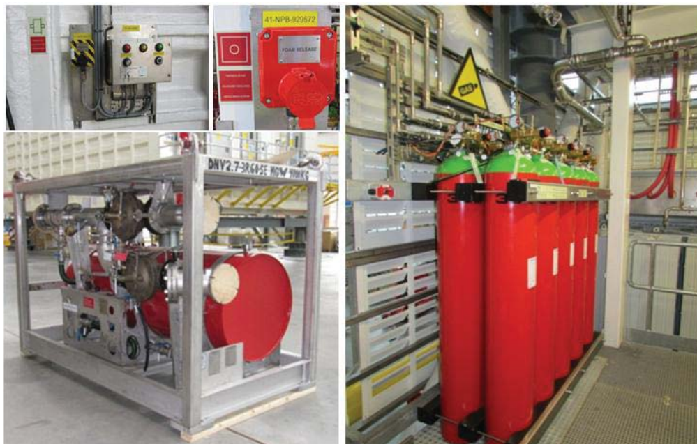
Safety Systems - Inergen and Foam
