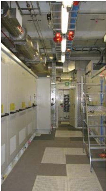
VSD Room Toward LV Room
