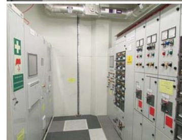
LV Room (SPCU,MCC,LV/UPS,HVAC)
